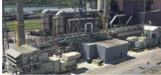
New Co-Generation facility Loudon, Tennessee
